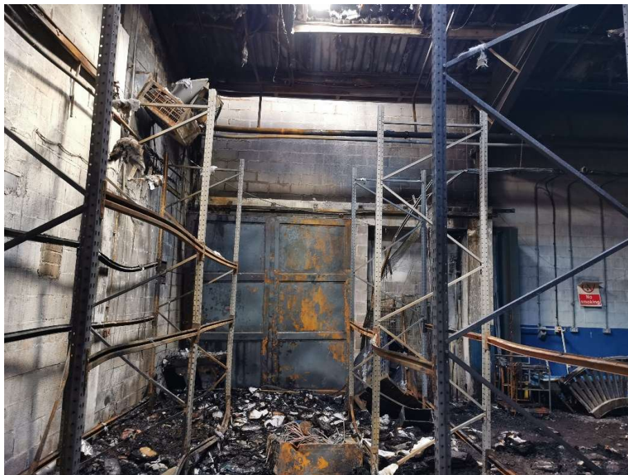
18. General overview of fire damage in Unit 2a.
