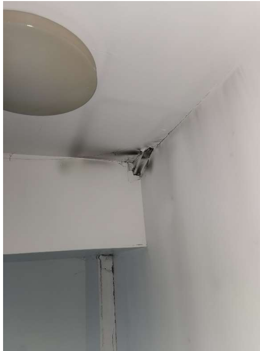
23. Smoke damage to staircase leading up to meeting room in Unit 2a.
