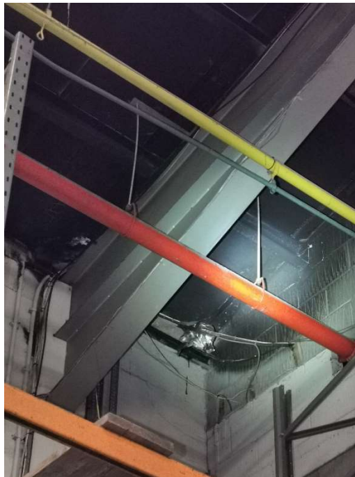
14. Smoke damage to roof in Unit 3.
