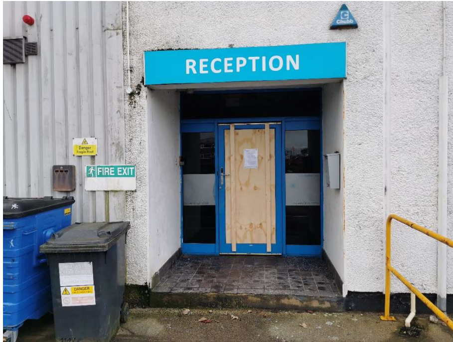
3. Damaged door to Unit 2b.
