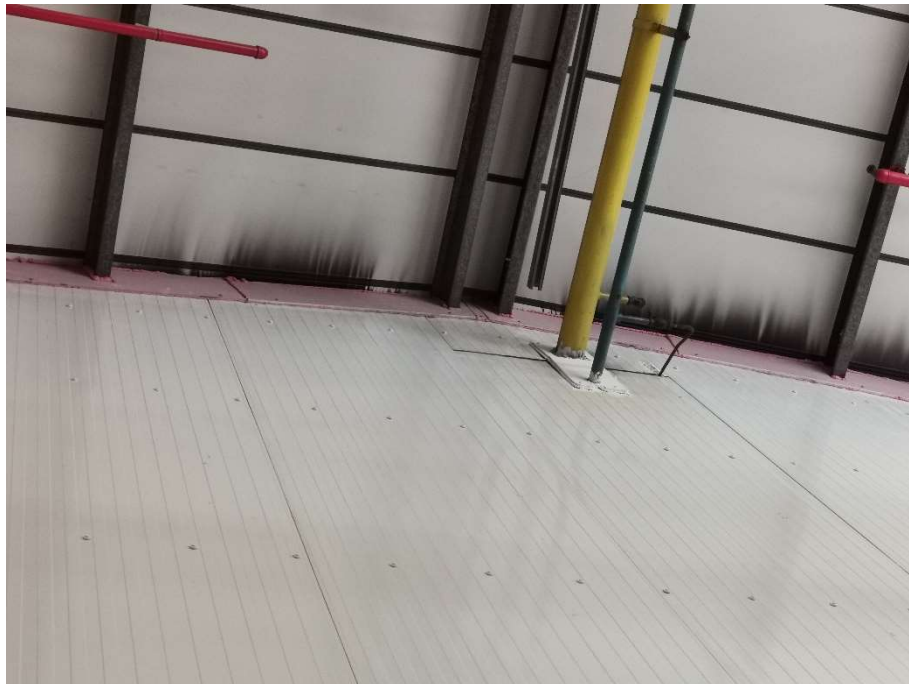
26. Smoke damage to the underside of the roof to Unit 1 at the party wall junction with Unit 2a.
