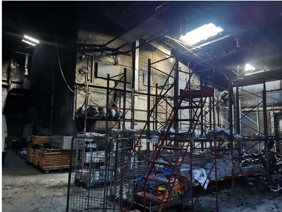
17. General overview of fire damage in Unit 2a.
