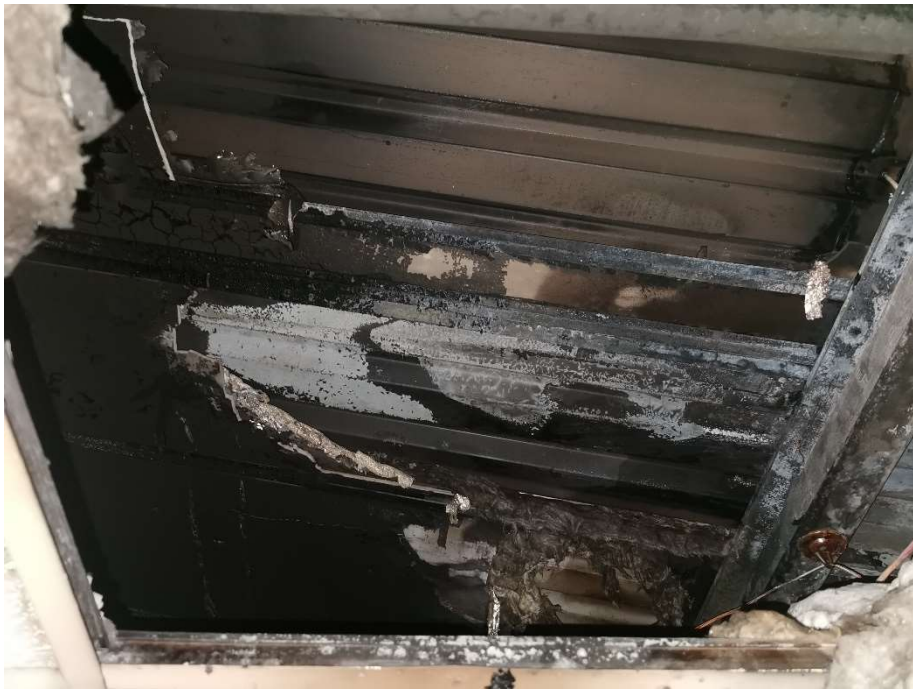
12. Server room at first floor level within Unit 2b.
