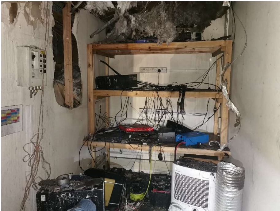
10. Server room at first floor level within Unit 2b.
