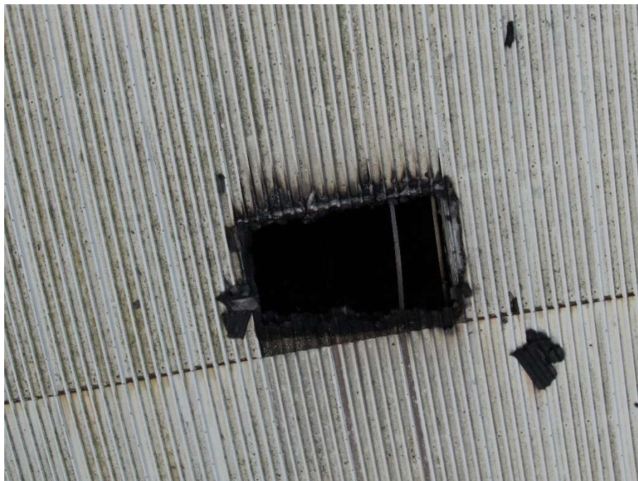
8. Fire damaged caused to the roof.
