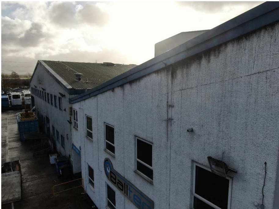
6. Smoke damage below the verge trim.
