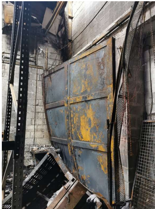
20. General overview of fire damage in Unit 2a.
