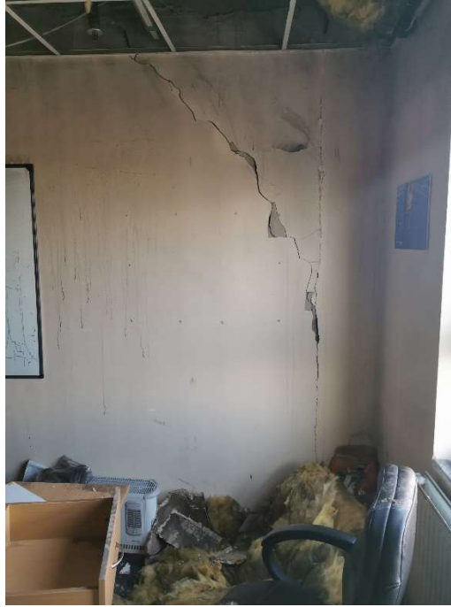
13. Cracking to part wall between units "a and 2b.
