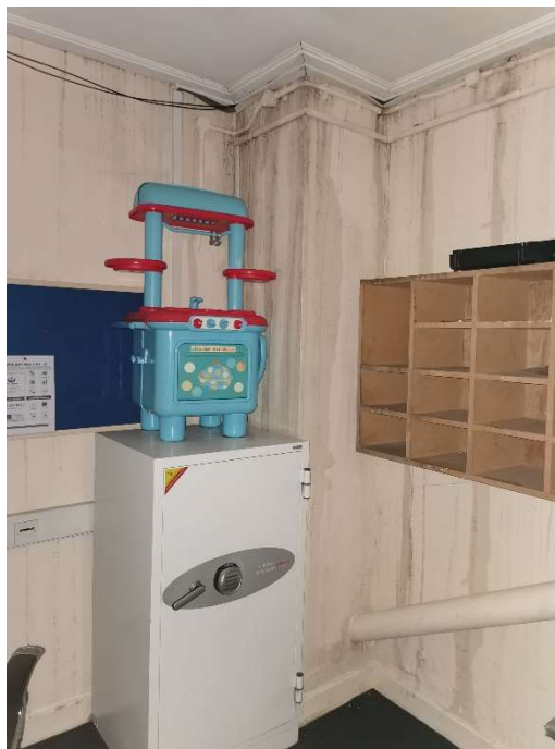
16. Water and smoke damage to Unit 2b at ground floor level.
