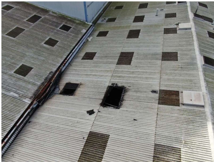
4. Overview of roof showing damage caused by the fire.
